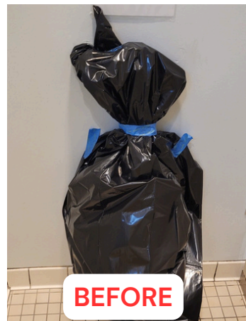
Fitness Center Broken Men's Urinal Replaced & Painted at Fitness Center -RMS & GMS
