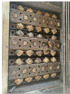
Heat Plates Before
