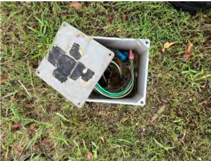
Area 9 Assigned To Maintenance Cover was placed back on top but a few screws are needed to secure the cover
