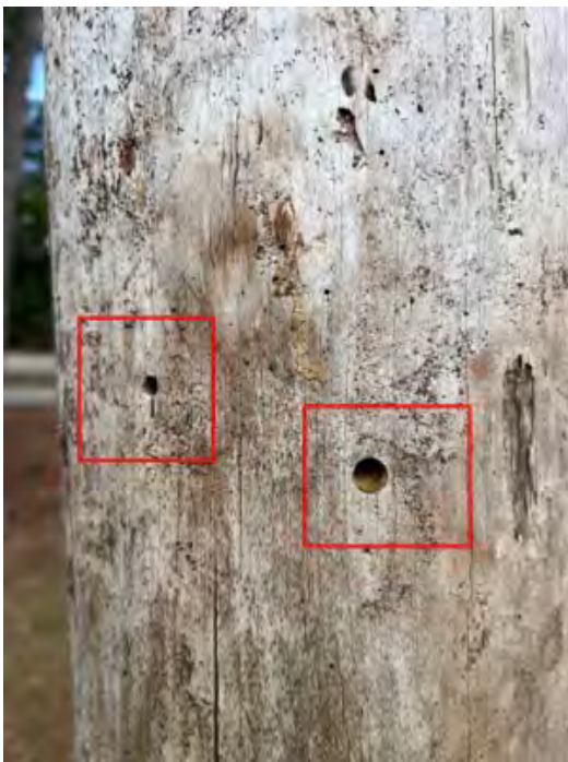
Area 17 Possibly pine bark beetle boring into pine trees. Inspect and propose a treatment that can help if they are present or to help prevent future spread
